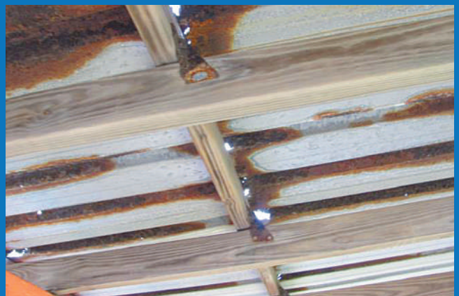
■ CORRODED ROOF SHEETS
