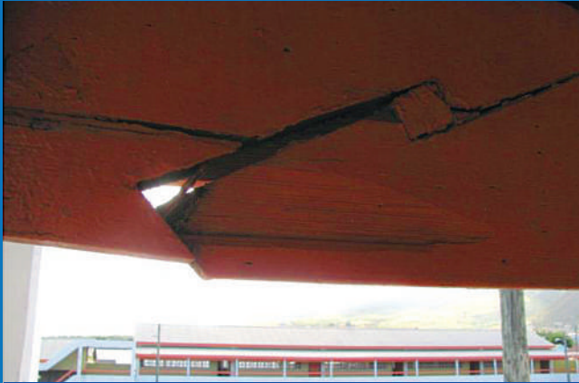
■ ROOF STRUCTURE IN A STATE OF DISREPAIR
