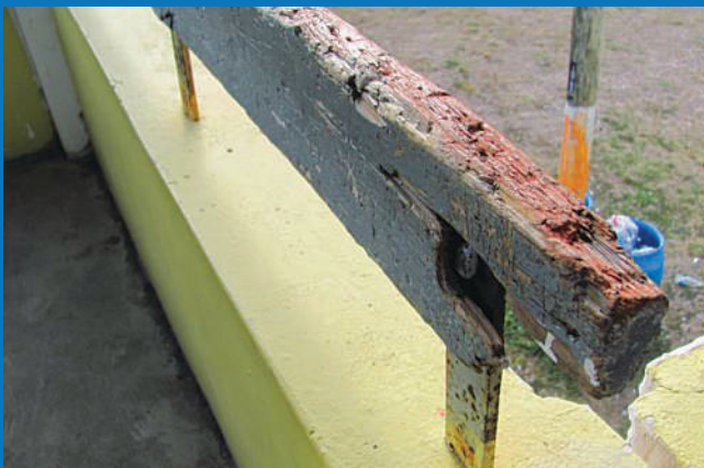
■ RAIL IN A STATE OF DISREPAIR
