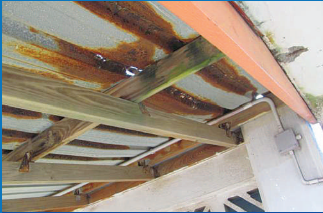
■ CORRODED ROOF SHEETS
