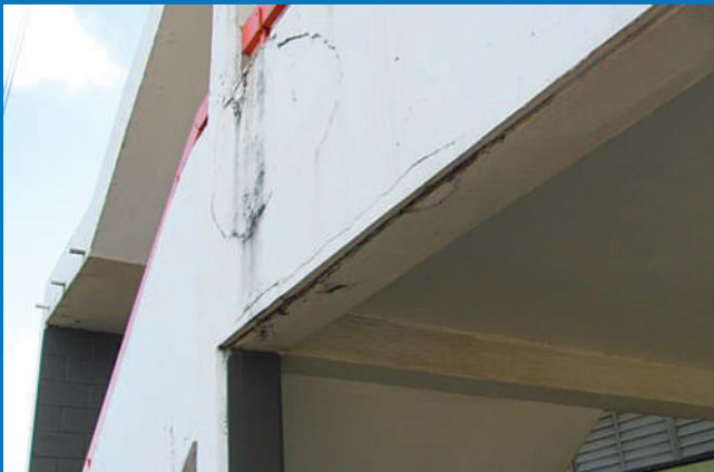
■ SPALLING CONCRETE - FLOOR BEAM
