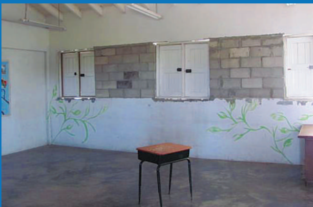
■ WINDOWS REPLACED WITH CONCRETE BLOCKS
