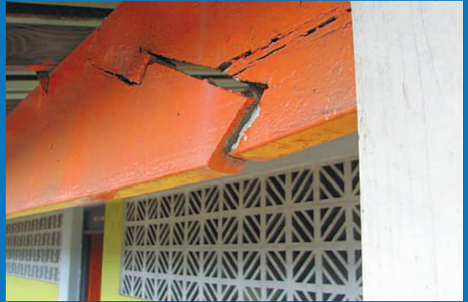
■ ROOF STRUCTURE IN A STATE OF DISREPAIR
