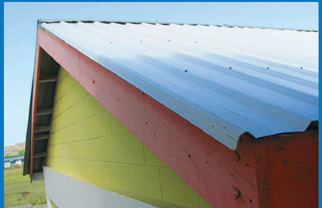
■ ROOF SHEETS WITH INADEQUATE SCREWS
