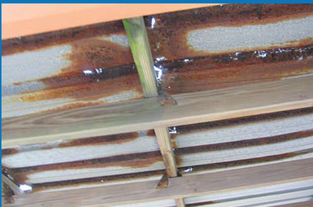
■ CORRODED ROOF SHEETS
