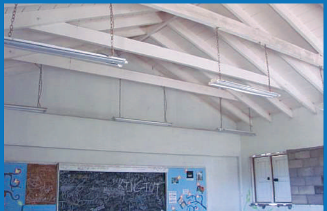
■ EXAMPLE OF LIGHT FIXTURES IN CLASSROOM
