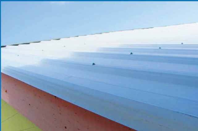
■ ROOF SHEETS WITH INADEQUATE SCREWS
