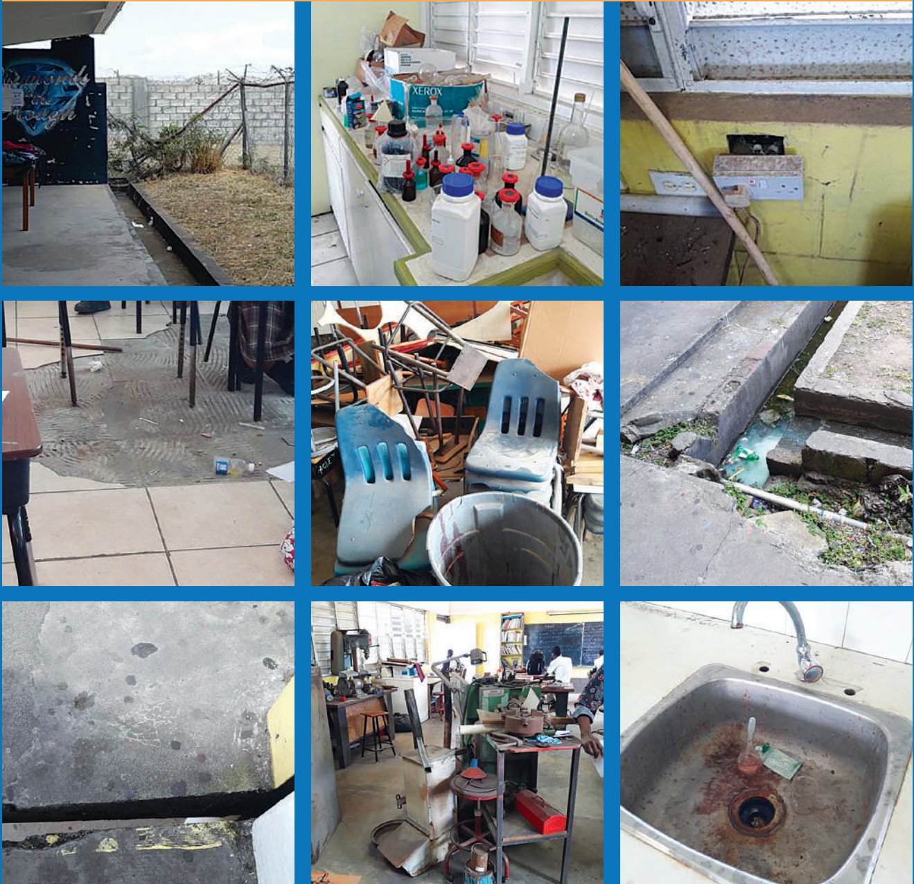
FIGURE 7.2: AREAS FOR IMPROVEMENT IDENTIFIED
