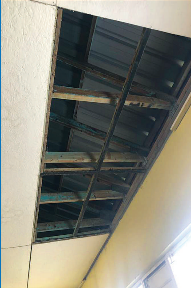
■ CEILING IN A STATE OF DISREPAIR
