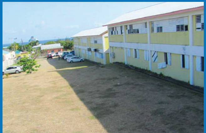
■ ELEVATION SHOWING WINDOWS IN A STATE OF DISREPAIR
