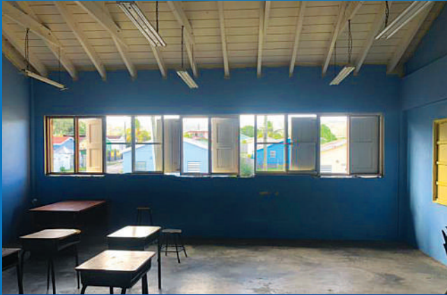
■ EXAMPLE OF LIGHT FIXTURES IN CLASSROOM
