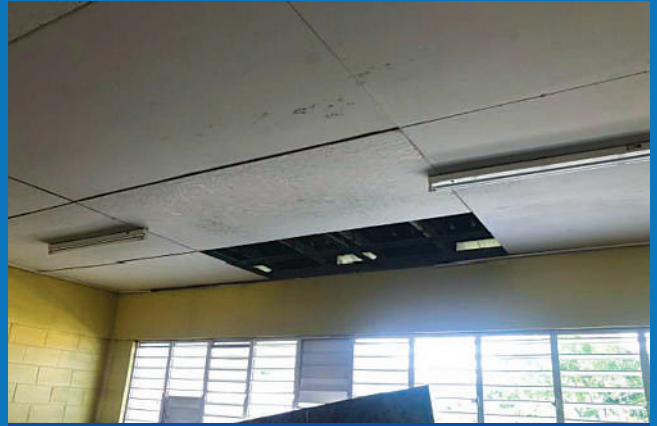
■ CEILING IN A STATE OF DISREPAIR
