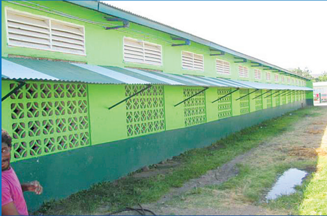
■ MAKESHIFT RAIN AND SUN SCREENS OVER VENT BLOCKS
