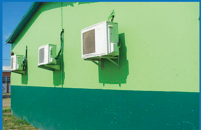
■ A/C UNITS INSTALLED FOR SPECIALISED ROOM
