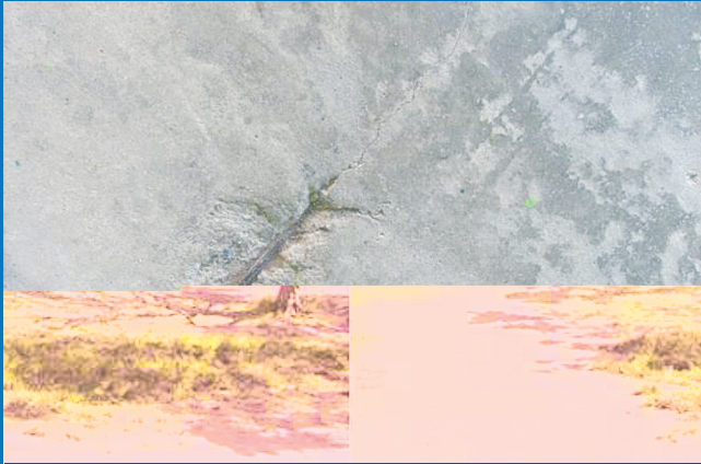
■ FLOOR SLAB TO BE REPAIRED
