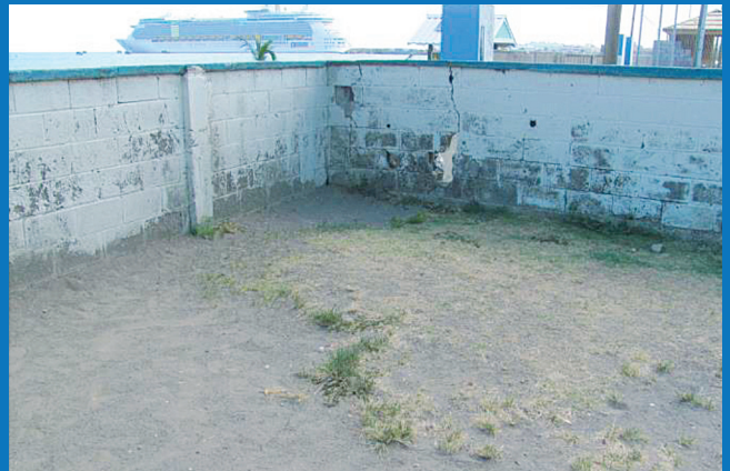
■ FENCE WALL IN A STATE OF DISREPAIR
