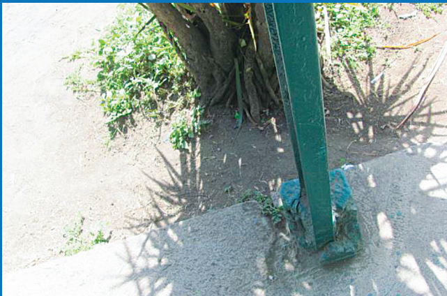
■ STANCHION SUPPORTS IN NEED OF REPAIRS
