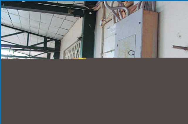
■ ELECTRICAL PANEL IN CLASSROOM
