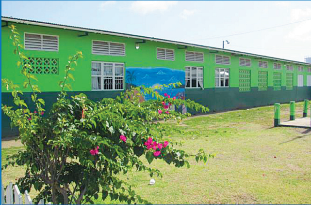
■ BLOCK WITH 3 DIFFERENT TYPES OF OPENINGS: GLAZED WINDOWS, FIXED WOODEN LOUVERS AND CONCRETE VENT BLOCKS
