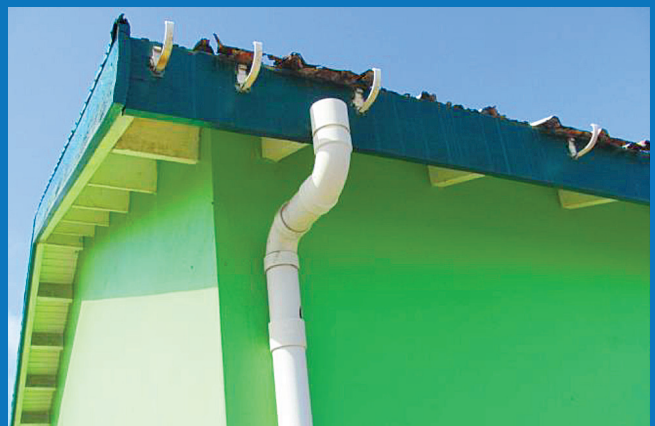
■ MORE RECENT BLOCK WITH GLAZED WINDOWS AND CORRODED ROOF SHEETING
