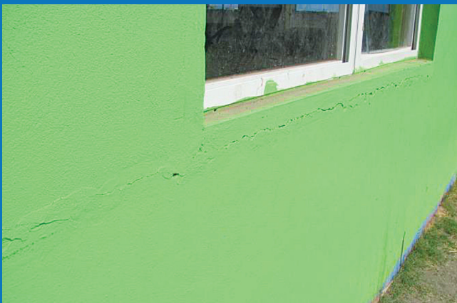
■ RECENTLY REPAIRED HORIZONTAL CRACKS
