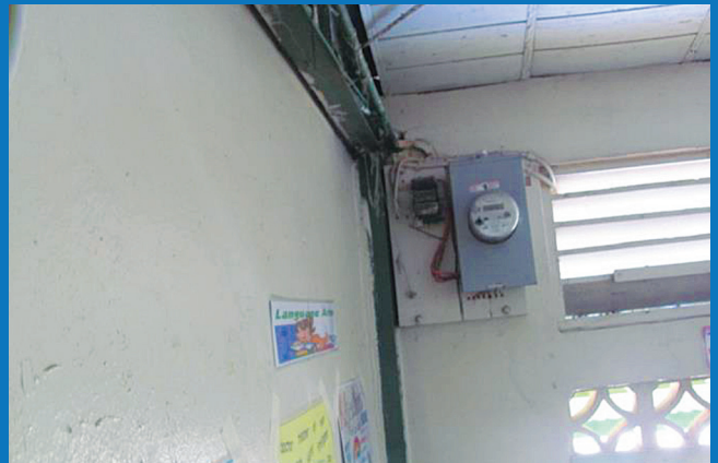
■ ELECTRICAL PANEL IN CLASSROOM
