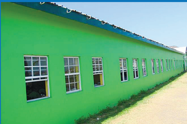
■ MORE RECENT BLOCK WITH GLAZED WINDOWS AND CORRODED ROOF SHEETING
