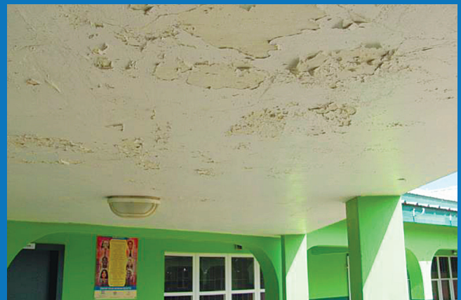
■ PEELING PAINT - INDICATIVE OF MOISTURE PENETRATION
