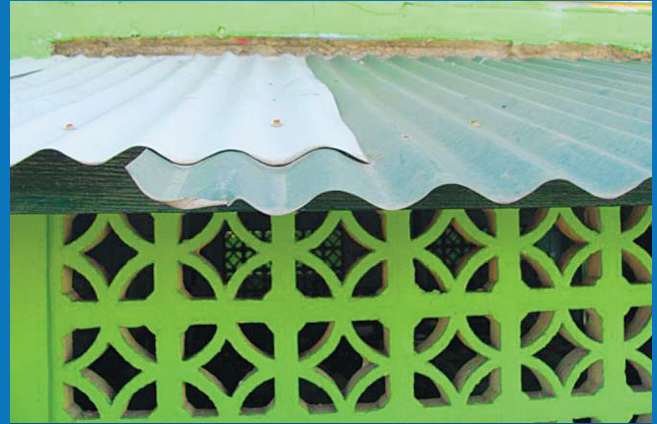
■ MAKESHIFT RAIN AND SUN SCREENS OVER VENT BLOCKS
