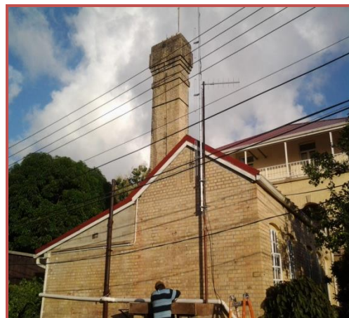
Figure 1: Installed antennas, SLARC project
