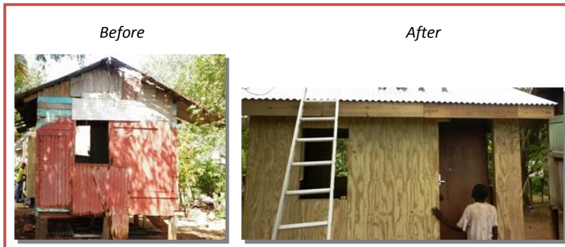
Figure 1: Repairs on a home in Telescope, St. Andrews (Grenada Red Cross Project)
