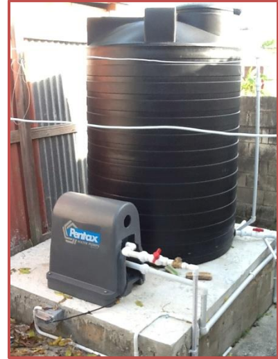
Figure 1: 400-gallon water tank and pump of a beneficiary of the MSSB project
