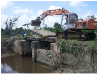
Crane preparing to lift sluice (flood) gate into position at the Sanica Sluice.
